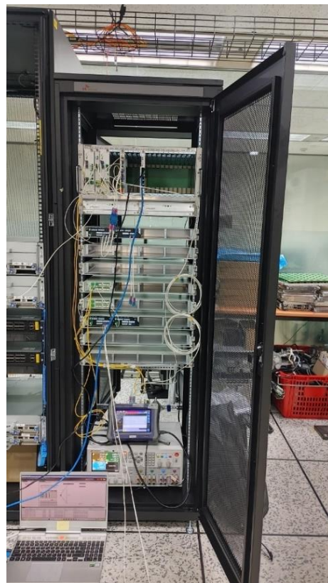
Figure 4 Photograph of the PoC rack in SK Telecom's 5G Lab
