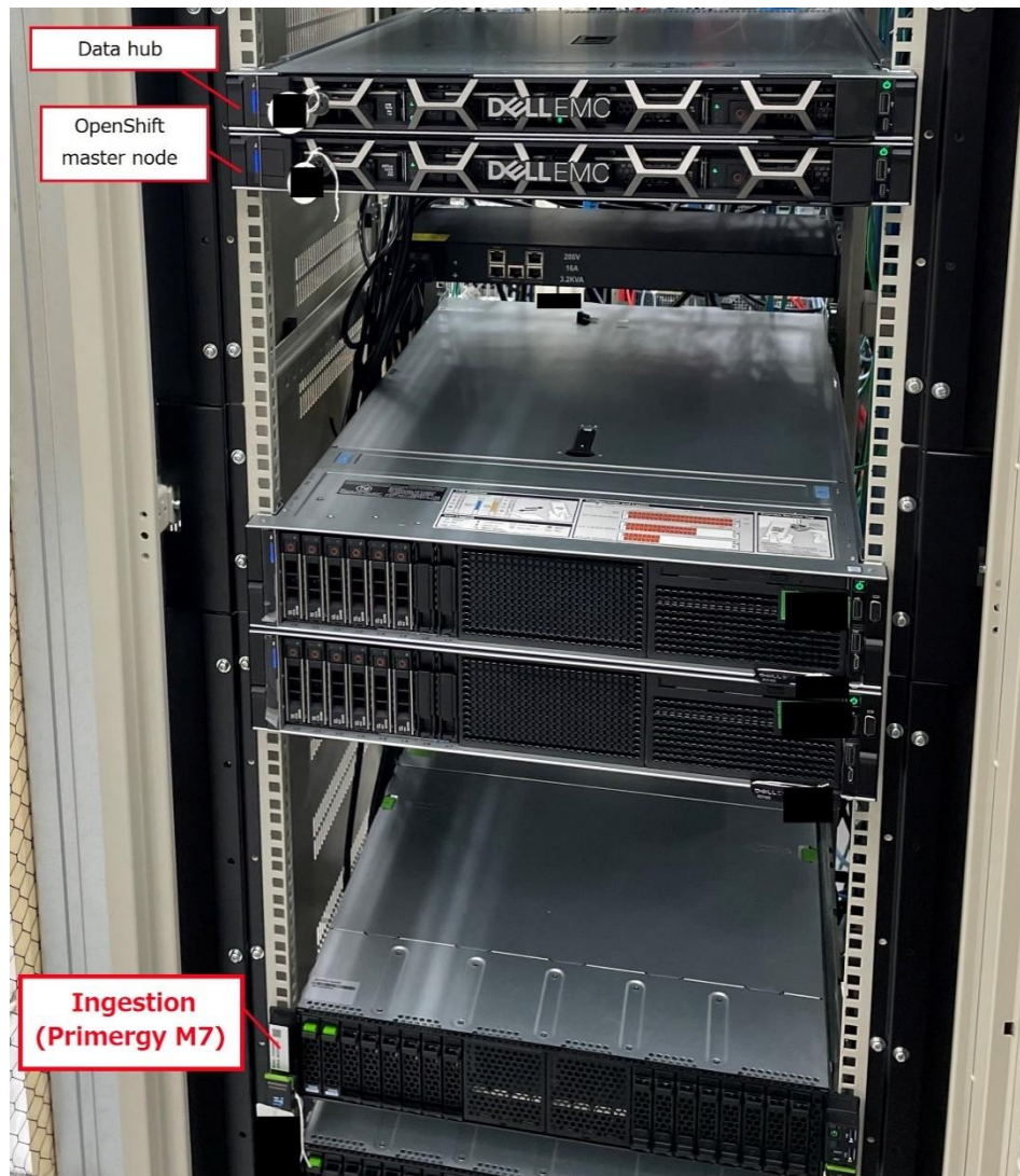
Figure 5-3: The ingestion node and the data hub node located in NTT Musashino R&D Center
